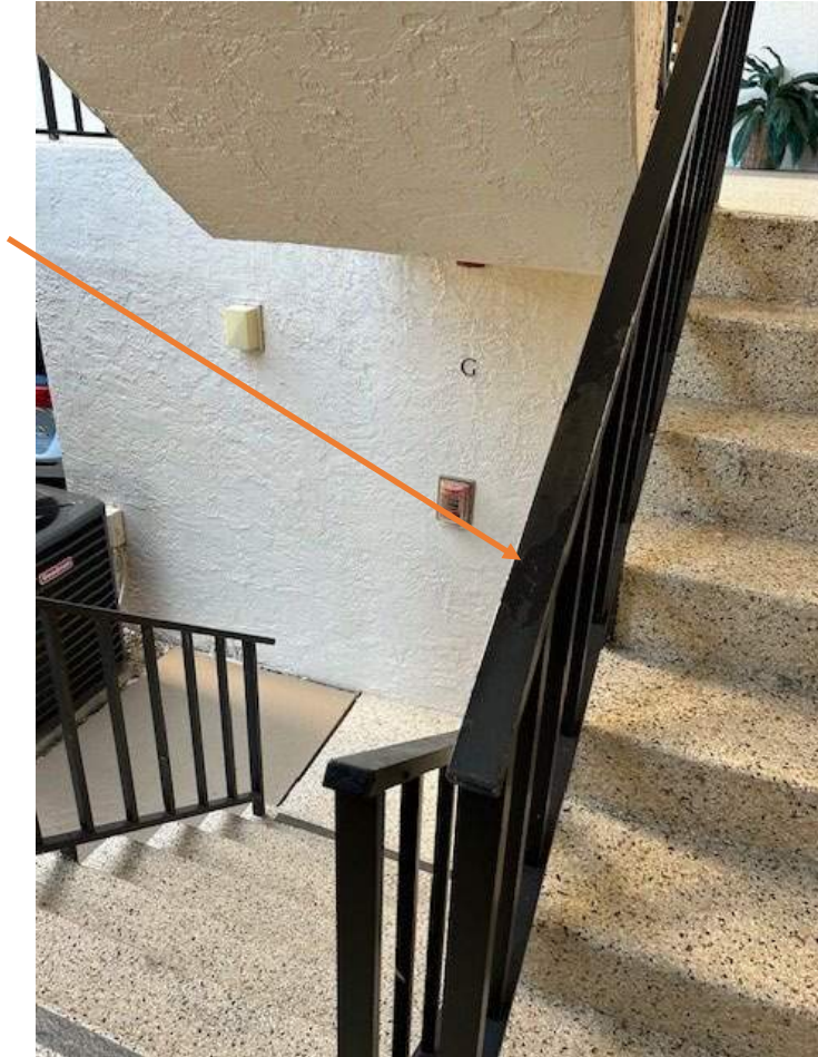
Figure 1: Peeling paint on handrail typical
