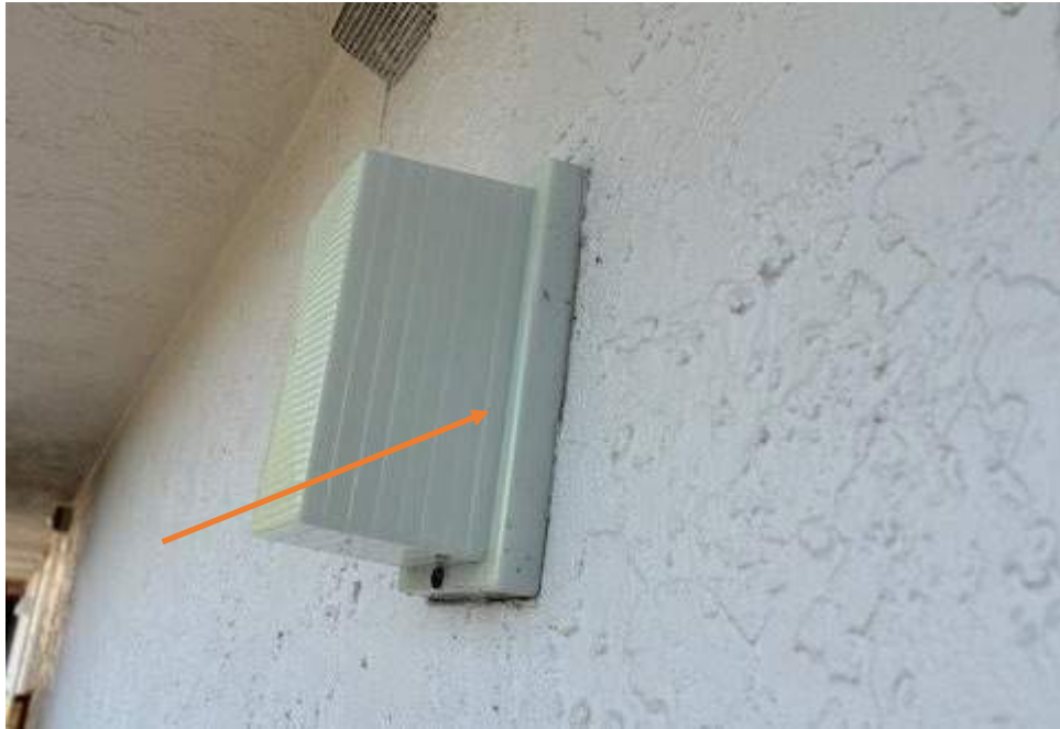
Figure 2: No sealant around light fixtures. Inspect foam seal regularly. Apply sealant if necessary
