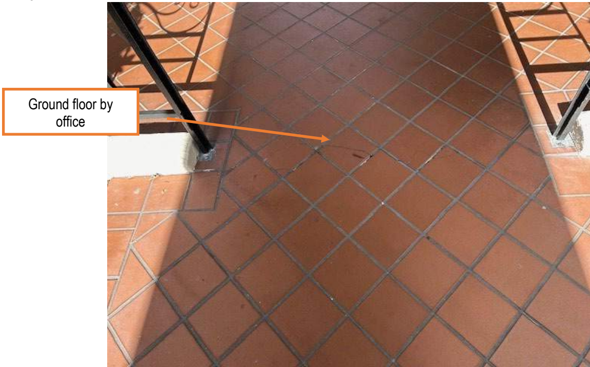
Figure 6: Cracked walkway tile
